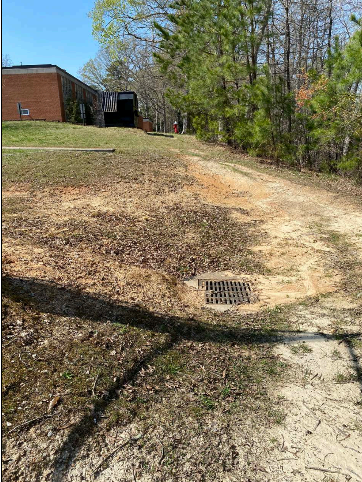
OF-11 (Photo 1 of 2) – Areas around the tennis courts are not stabilized, allowing potential for sediment to be transported via the storm sewer to the creek.
